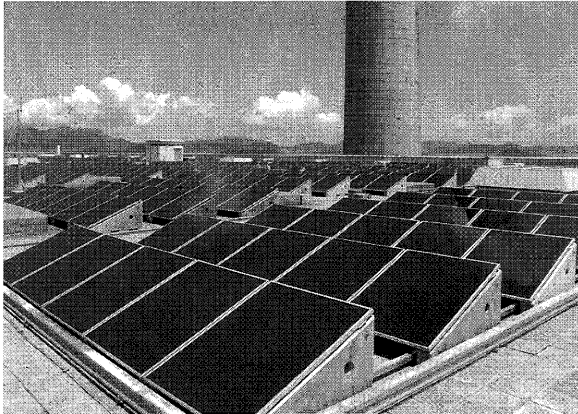
Figure 15 Completed PV System
