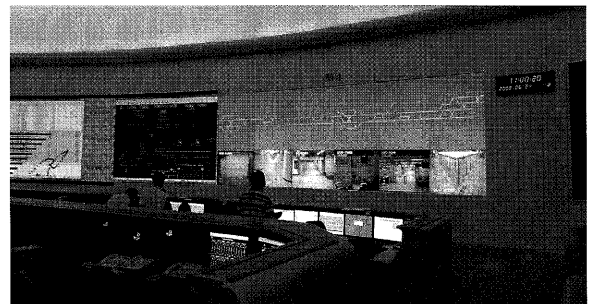
Figure 10 OCC During Commissioning
