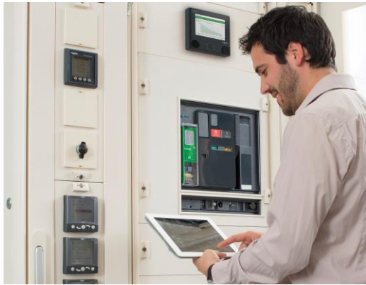
Fig. 2 – Smart, Connected Devices are the First Step in a Completely Digitalized Power Distribution System
