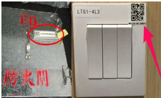
Fig. 3 – Examples of the Installation of RFID Asset Tag and Zonal QR Code
