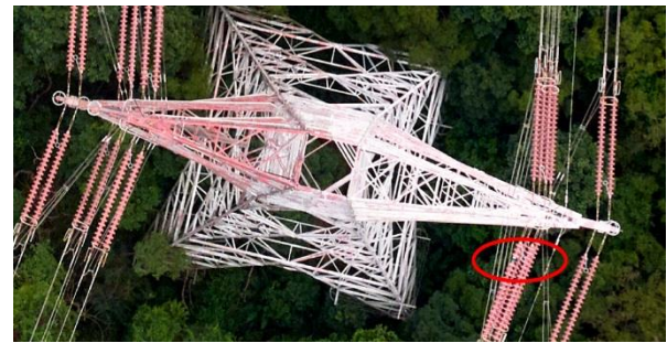
Fig. 9 – Insulator Condition Assessment – Broken Insulator Identified
