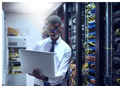
Fig. 1 – Facility Teams for Large and Critical Buildings need to Maintain the Safety, Reliability, Efficiency, and Compliance of their Electrical Infrastructures
