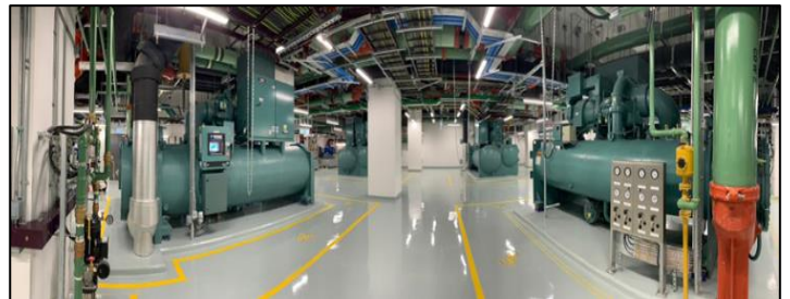
Fig. 26 - MiMEP Zero Welding Chiller Plant with Full BIM Implementation
