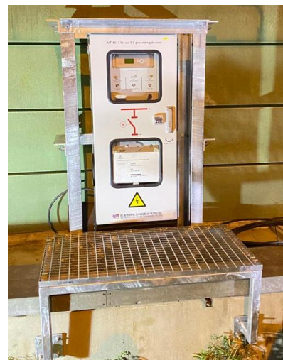
Fig. 7 - Remote Earthing Switch
