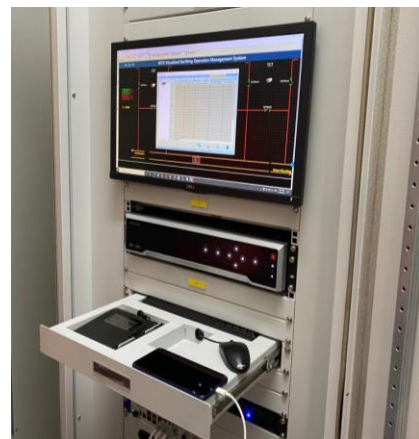
Fig. 13 - Control Console in Airport Station
