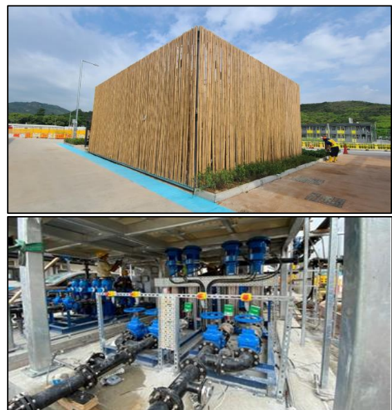
Fig. 23 - MiMEP Plant Room at Penny Bay
