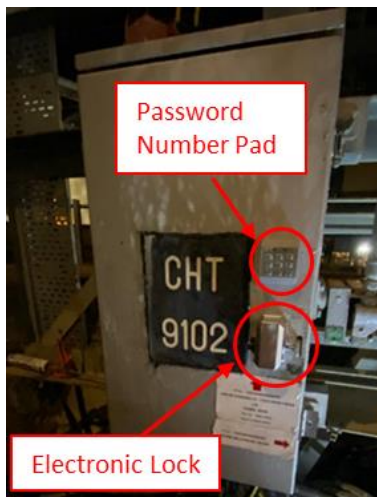
Fig. 9 - Modified OHL Isolator Control Cubicle with Electronic Lock and Password Number Pad
