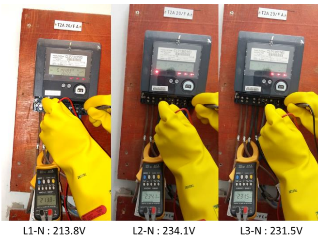
Fig. 13 - Voltage Readings are Verified during a Meter Inspection to ensure Proper Meter Operations
