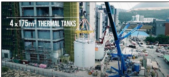
Fig. 29 - Mega Scale Tailor Made DfMA/MiMEP - Thermal Tank in a DfMA Project showcasing Better Safety Performance with Minimized Site Risk
