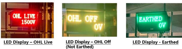
Fig. 10 - OHL Energization Status Display Panel
