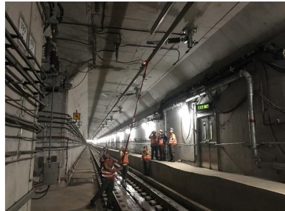
Fig. 1 - Existing Testing and Earthing of OHL
