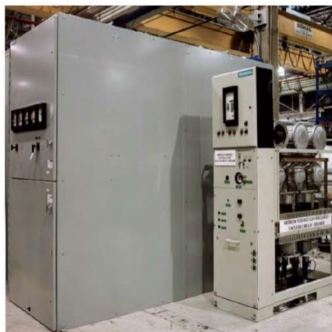
Fig. 1 - 36kV Indoor MV Switchgear Comparison (AIS on left, SF6 GIS on right). [2]
