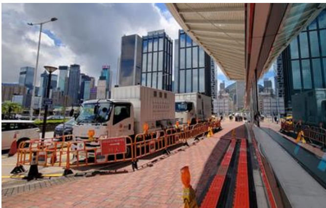
Fig. 13 - Use of EST and PCT to Maintain Supply Security of Important Event
