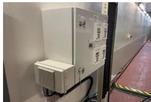
Fig. 4 - Cable Incipient Fault Detection System
