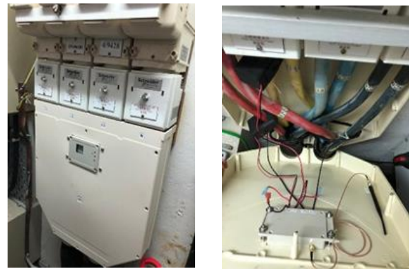
Fig. 11 - Inhouse Developed LV Fault Indicator and the Wiring Connection
