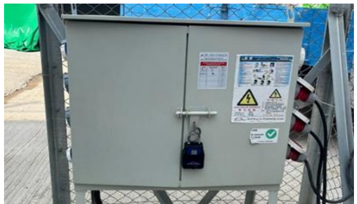
Fig. 9 - Smart Lock System for Electric Box Management
