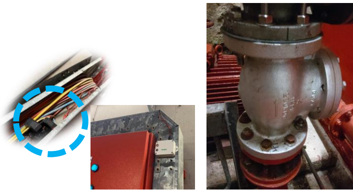
Fig. 9 - Monitoring Operation Current of Fire Service Pump
