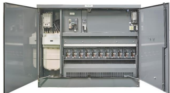
Fig. 2 - Typical Low-Voltage Assembly with Integral Tariff Metering Facility
