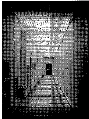
Figure 3 Natural Daylight Effect in Corridor of So Kwun Wat 132kV Substation
