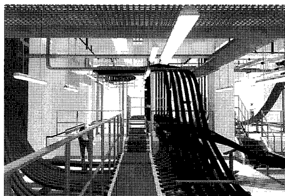
Figure 12 Future Layout of Cables inside Basement of Junk Bay Road 132kV Substation
