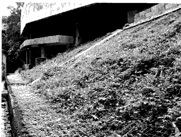
Figure 5 Seasonal Complementary Green Wall System at Chuk Yuen 132kV Substation
