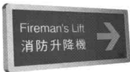
Figure 10 Fireman's Lift Direction Sign
